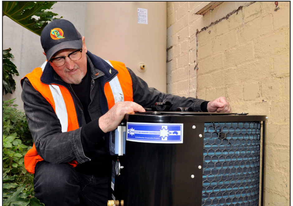
Hot stuff: Earthworker’s Dave Kerin checks over a hot water pump newly installed for community housing run by the Father Bob Maguire Foundation.
